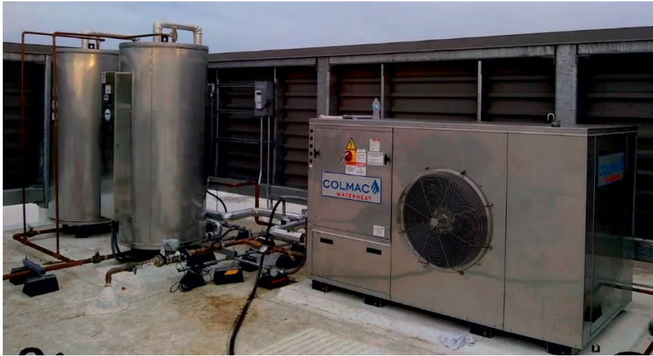
Large installations on roof are most common. Used with permission of Colmac WaterHeat.
