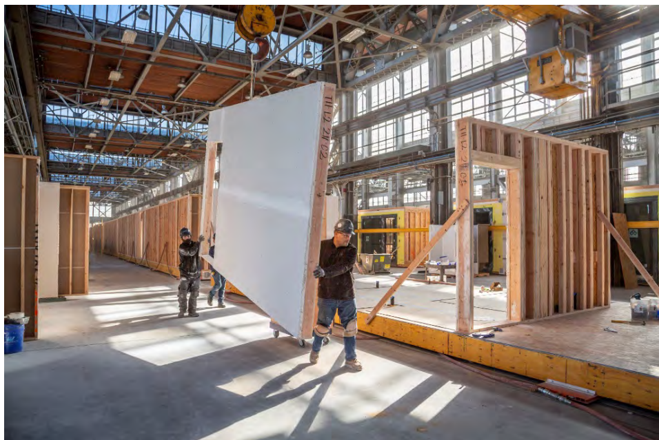
Wall assembly on the factory floor using gantry cranes. Image courtesy of Autodesk.
