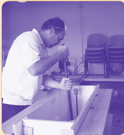
Student Harold Meckler is using an iron tamping tool to compact moist soil in a wooden form to construct a rammed earth wall.
