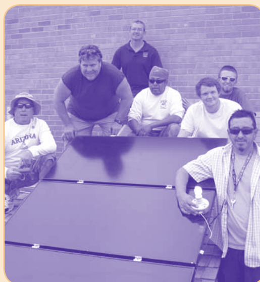
Students (left to right) Jeffrey Fagenbush, Kenneth Herbert, Rex Turvin, Cornelius Lewis, Max Bolt, Dallas Leavell, and Alex L'Esperance are proud of their solar panel mounting accomplishment.
