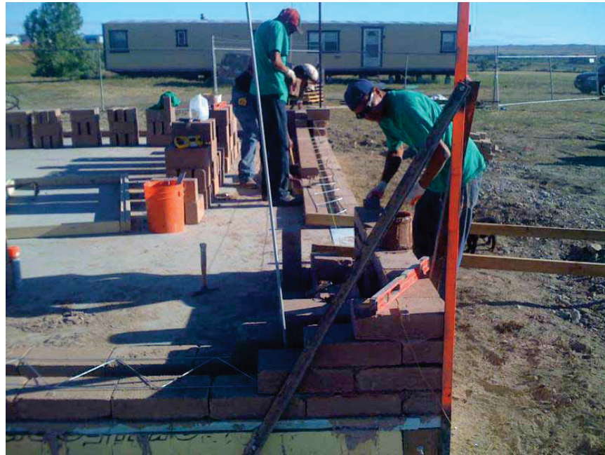
Figure 11. Orange Story Pole at Corner Bolted and Braced to Foundation
